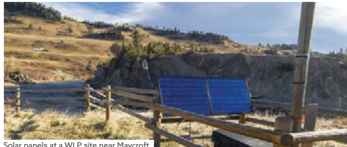
Solar panels at a WLP site near Maycroft.
